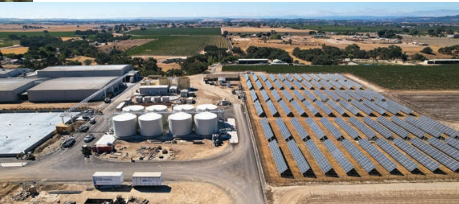
The J. Lohr team strives for continuous improvement. Pictured at the winery’s Home Ranch in Paso Robles are the foundations for two new cooperage buildings that will hold 32,000 barrels, eight new bottle-ready storage tanks, a nearly completed water-treatment system, solar panels that provide 75% of the winery’s power, and composting fields.
